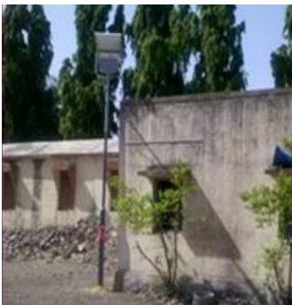
Solar Street Lamp at Hatnur Kannad, Aurangabad
